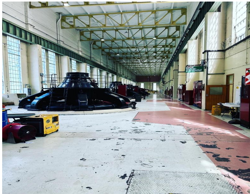
Figure 2: Captured By Me The Turbines Inside The Power Generation Room
