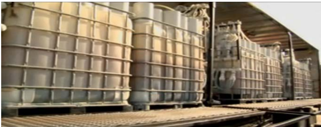
Figure 88 - Trailer mounted FO filtration system (EMERALDSURF,2008)
