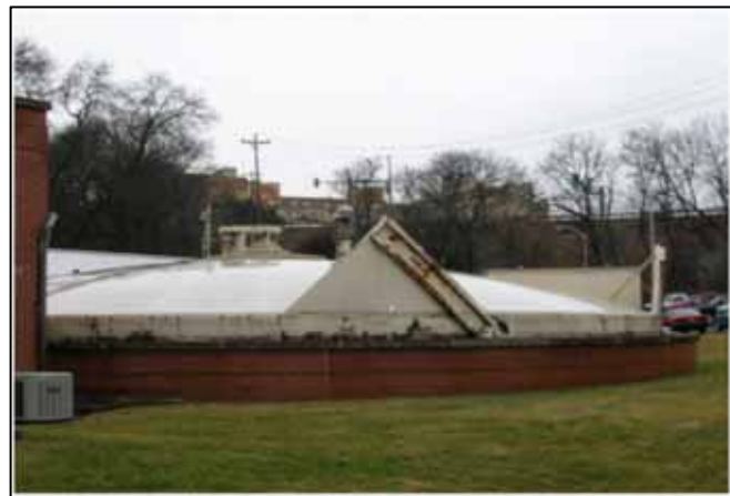
Fig. 8 Primary Digester at WWTP
