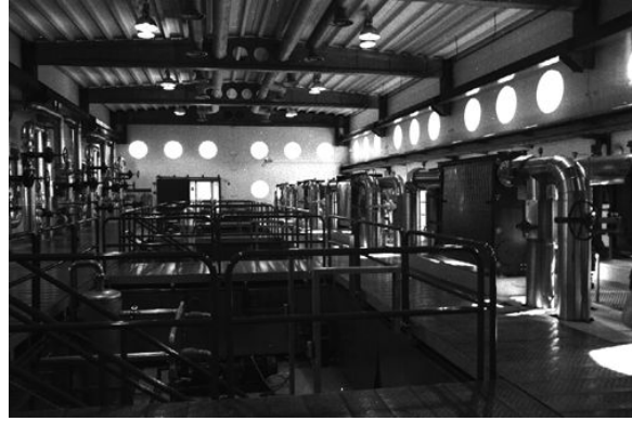
Figure 8: Geothermal power plant in Njardvik, Iceland. Photo by M. Narkiewicz, May 2003.
